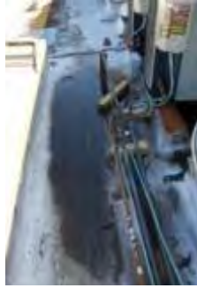
Signs of standing water/pooling
