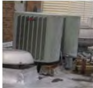
Trane condensing units
