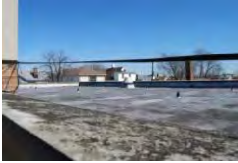
The roofing material has reached the end of its useful lifespan.
