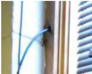
Un-caulked/un-sealed exterior wall penetrations
